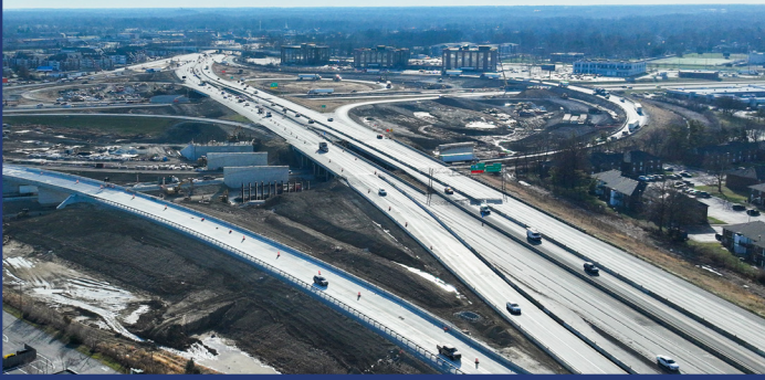
First new system ramp and bridge from I-69 South to I-465 West
